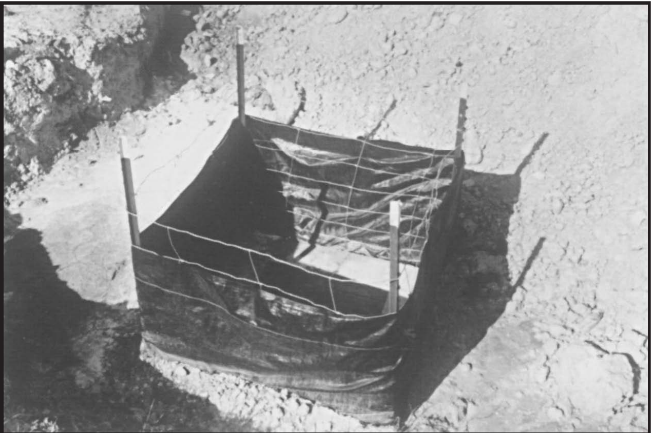
Figure 6.40 Filter fabric is only one way of protecting storm water inlets from siltation early in the grading process.
