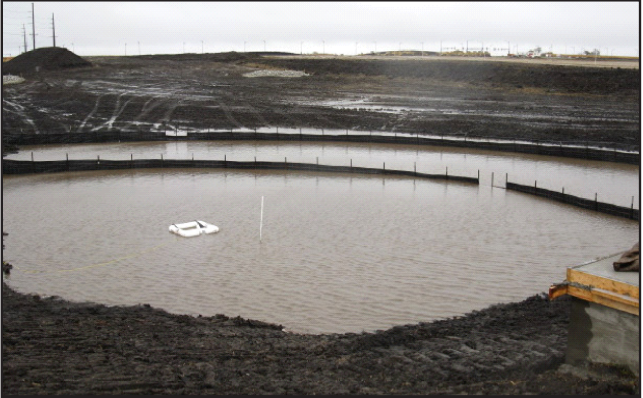
Figure 8.89 A sediment basin can be used to pretreat sediment-laden water before it discharges from the construction site. Source: BFA Inc.
