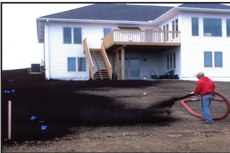
Figure 6.66 Applying a compost blanket in a new housing development. Source: Iowa Natural Resource Conservation Service, Urban Conservation Photo Gallery www.ia.nrcs.usda.gov/features/
