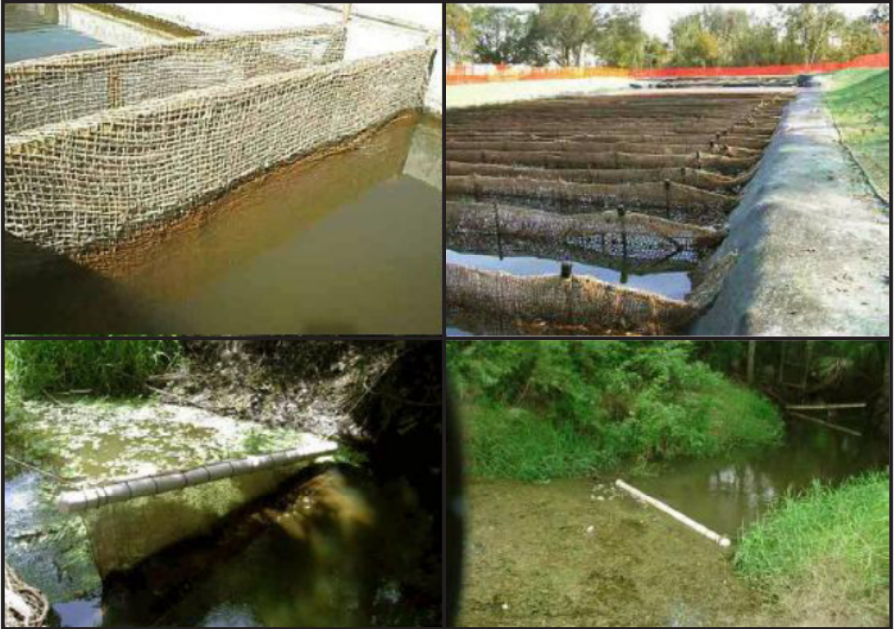
Figure 6.91 Particle Curtains. Source: Florida Erosion and Sediment Control Designer and Reviewer Manual, June 2007
