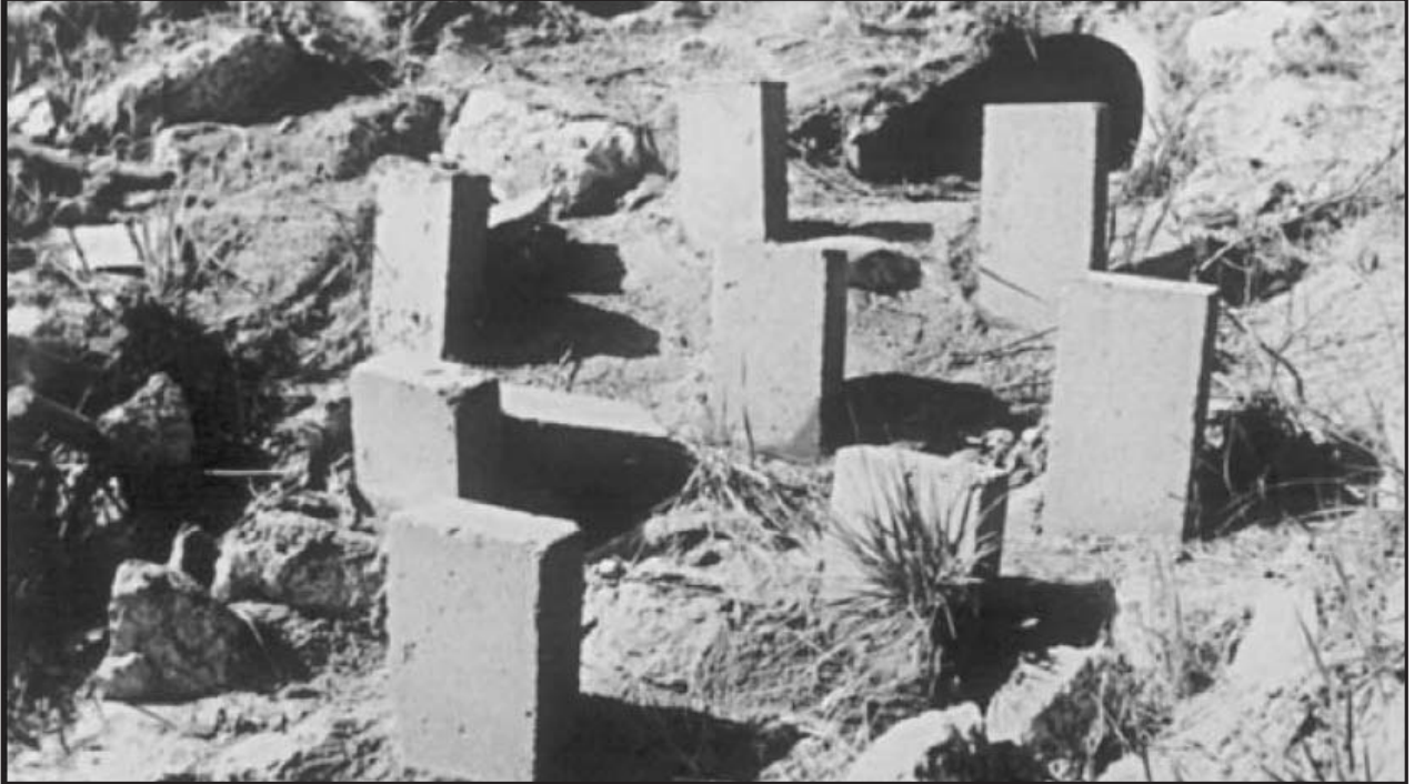
Figure 6.74 Energy dissipators reduce flow velocities so water can exit at nonerosive rates. Source: C. Rahm, NRCS St. Charles Co.
