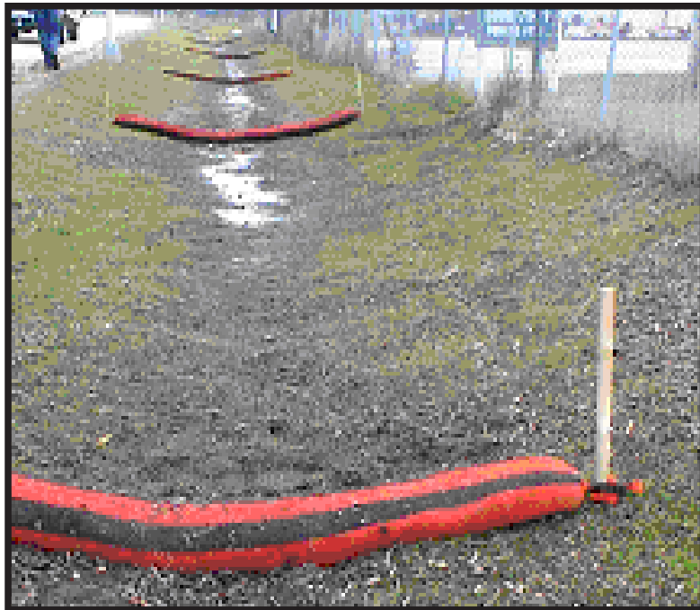
Figure 6.70 Installation of filter socks in a road ditch by Indiana Department of Transportation. The filter socks will be staked through the center. Source: EPA NPDES Stormwater Menu of BMPs, Compost Filter Socks .
