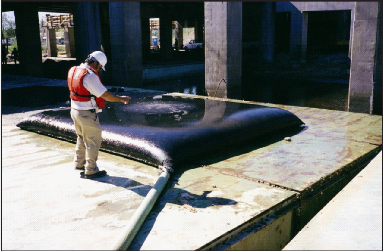
Figure 6.88 Use of a dewatering bag where storm water is pumped into a geotextile bag. The sediment stays in the bag while the storm water is allowed to flow out through the small voids in the material. Source: ACF Environmental Inc.
