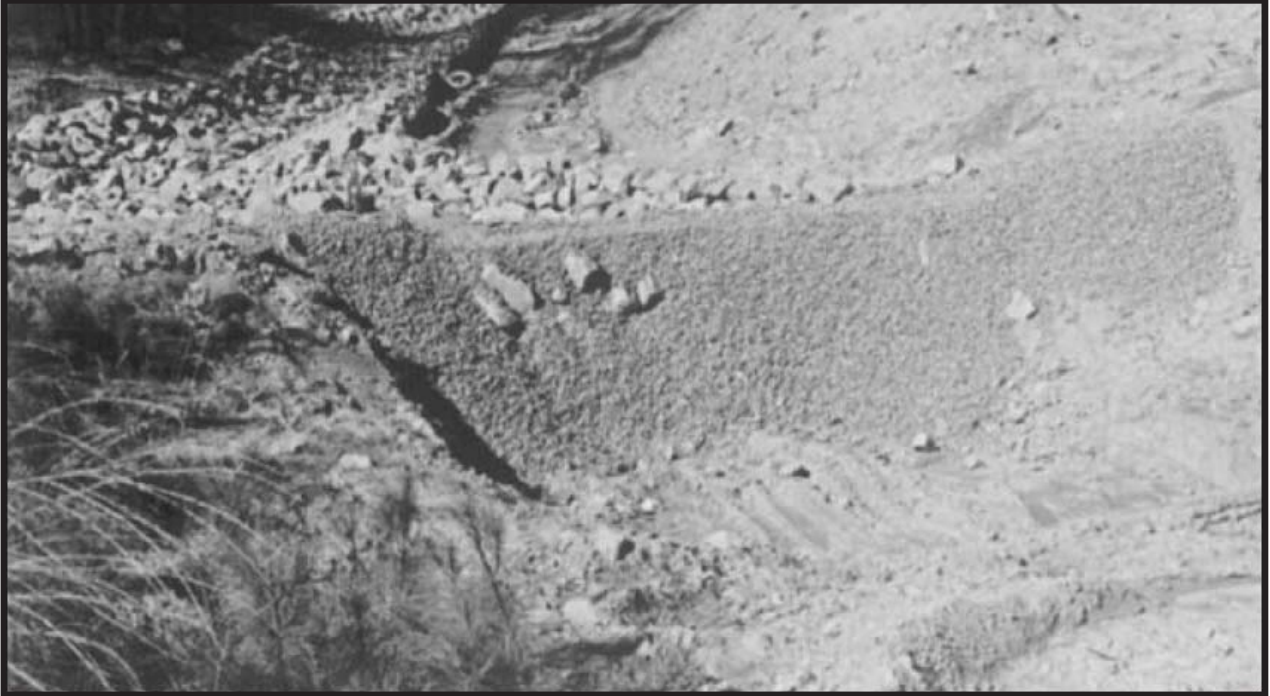
Figure 6.79 Rock check dams can provide sediment control in channels and swales. Source ABC of BMPs, LLC
