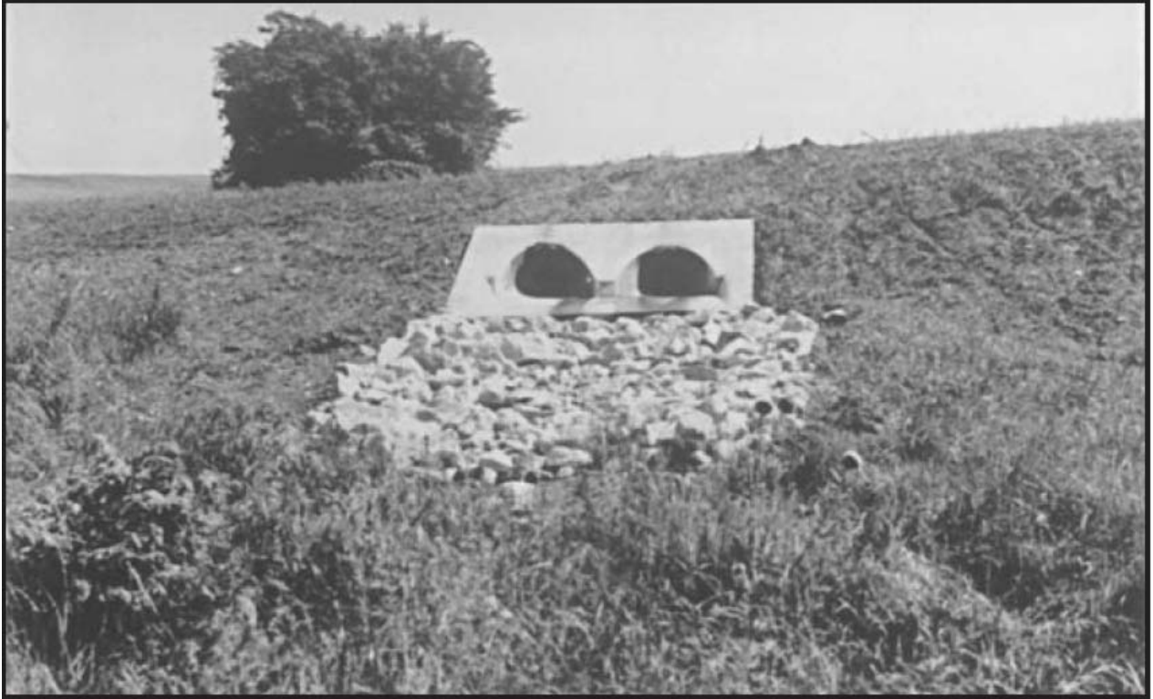
Figure 6.64 Riprap at the downstream end of a rock outlet should be level with the receiving channel or slightly below it . It should not restrict the channel or produce an overfall that will result in scouring and erosion. Source: Becky Holland, NRCS Volunteer. Jackson Co.
