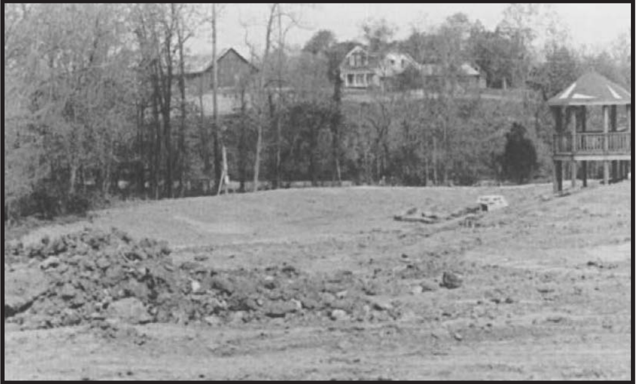
Figure 6.55 An unfinished temporary diversion routes sediment-laden storm water to a sediment basin. Temporary diversions should be shaped and protected with a turf reinforcement mat or rock. Establish permanent vegetation if the diversion will be used for one year or more. Source: K. Grimes, Soil and Water Conservation District, St. Charles Co.
