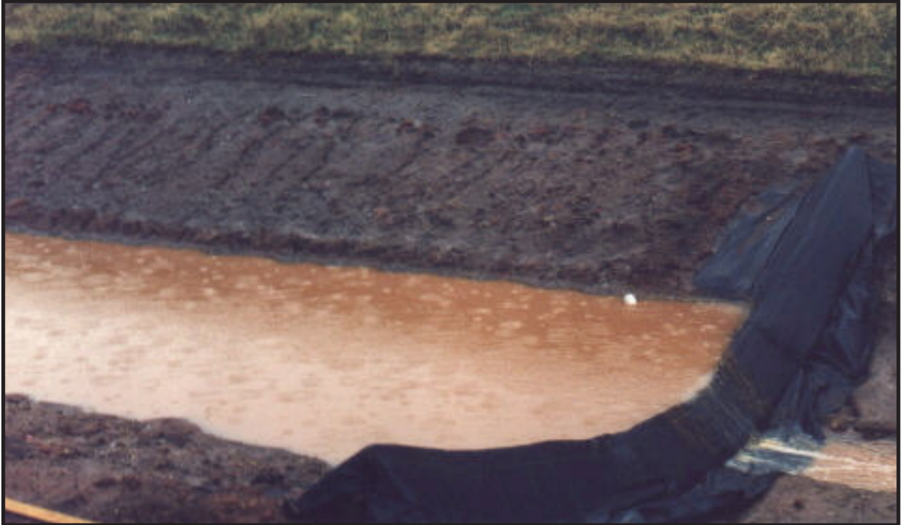
Figure 6.81 This check dam device appears to be working correctly but there should also be erosion control protection covering the channel to reduce scour and erosion of the channel bottom. Source ABC of BMPs, LLC
